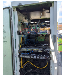
Deployment at Company owned Solar site (MA)
