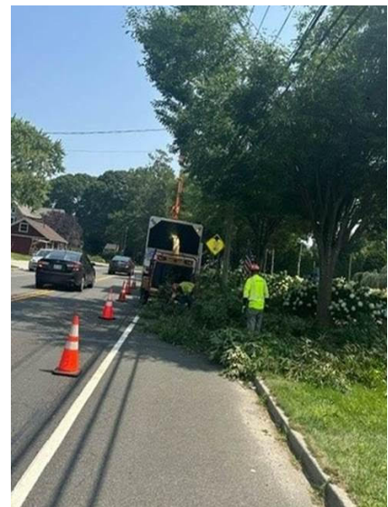
Figure 9. Completion of pruning to create a buffer between the power lines and nearby trees, reducing outage threats.
