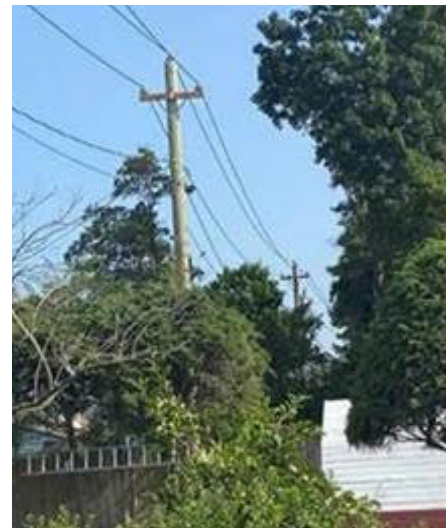
Figure 2. A storm-hardened distribution circuit.
