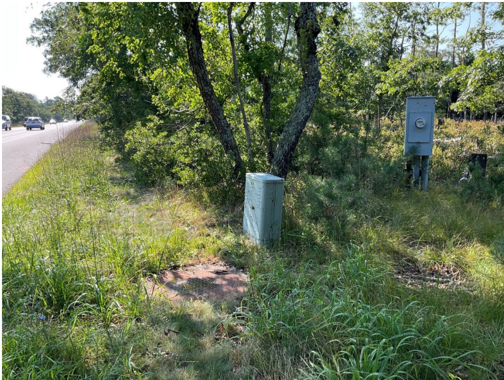
Photograph A-18. View of manhole cover and electrical boxes (and meter) on southern side of Route 114; write-off area (Chronicle Heritage, August 2024).
