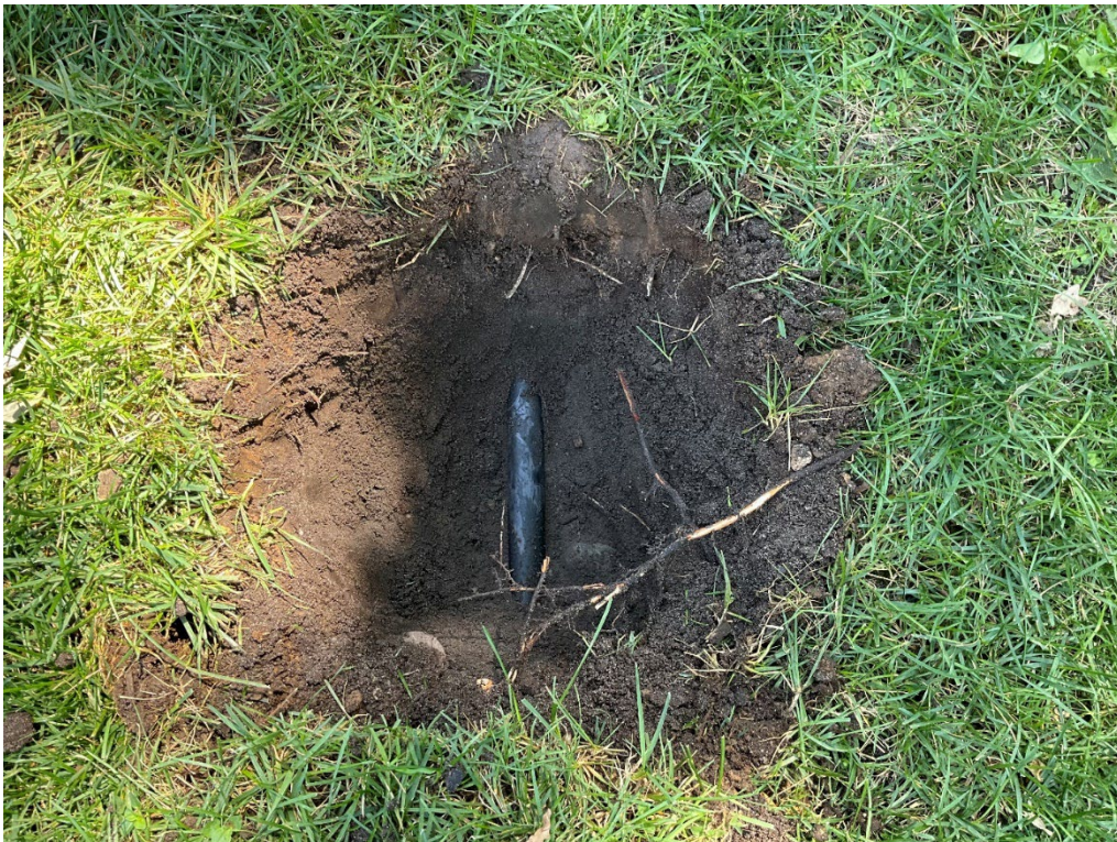
Photograph A-12. Example of cable utility exposed in STP 103 (Chronicle Heritage, August 2024).
