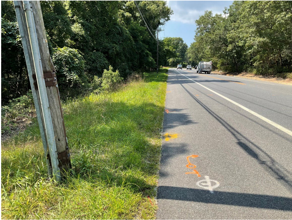
Photograph A-13. View of gas and telephone utilities on southern side of Route 114, west of Goodfriend Drive (Chronicle Heritage, August 2024).
