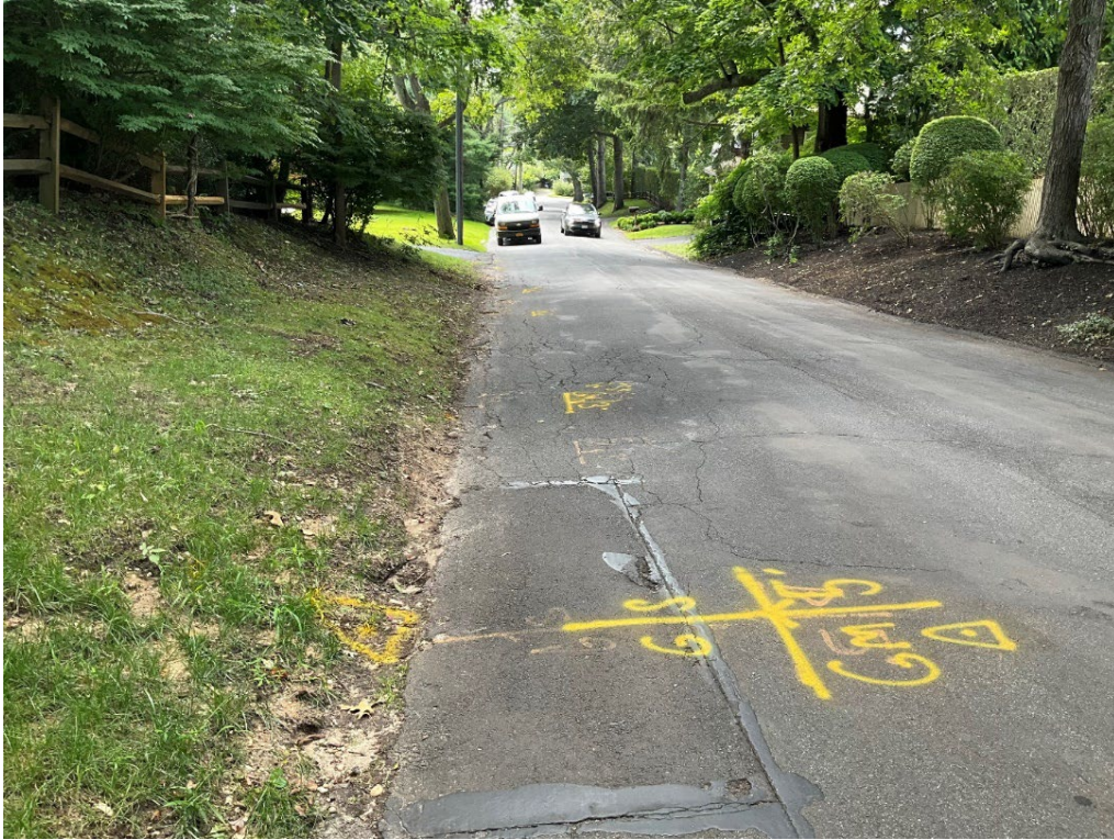
Photograph A-7. Southern side of Harrison Street with utility mark-outs showing buried gas line (Chronicle Heritage, August 2024).
